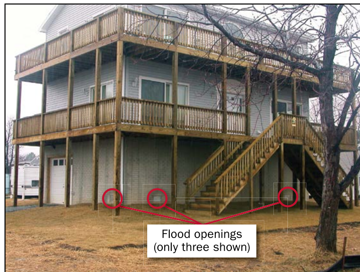
Figure 3: Full-height, solid perimeter walls surrounding a garage and storage area with flood openings (only three openings are shown)
